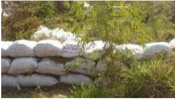
Fig2. Earthen and bori bunds/sand bag checkdams
